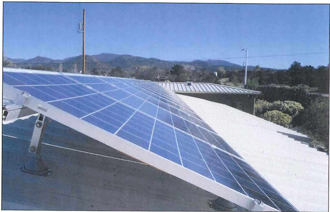
The rooftop solar array at Santa Fe Girls' School
